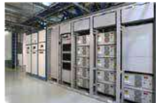
Wyndham Data Centre
